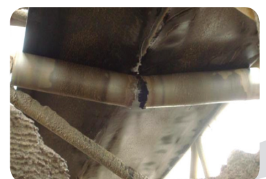
Failed Steel Roll results in costly belt rip and conveyor downtime.
